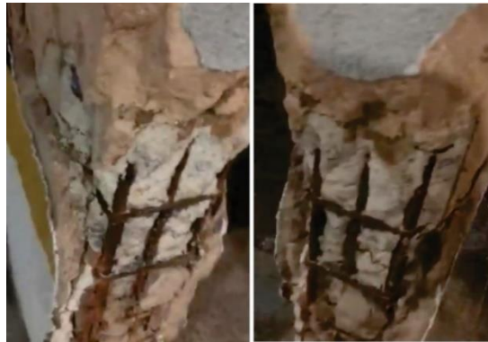
Figure 1 – Exposed column reinforcements
